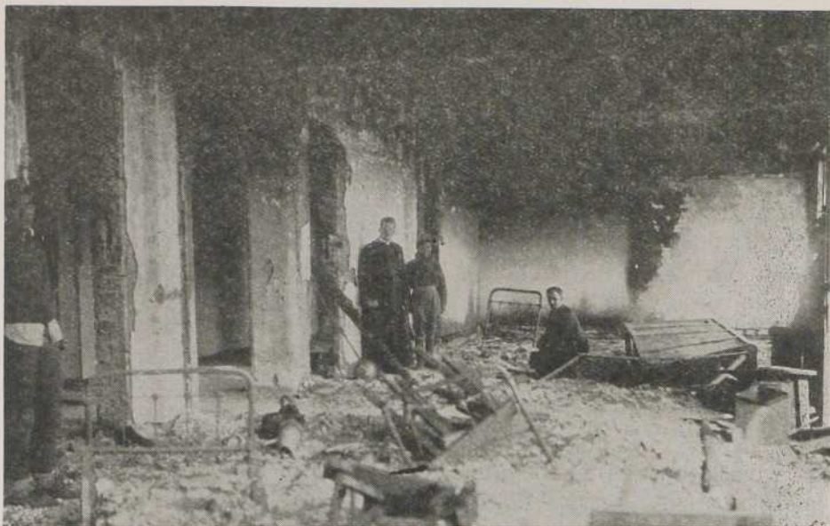
SZEPINGKAI SEMINARY. DAMAGES CAUSED BY AN INCENDIARY BOMB
